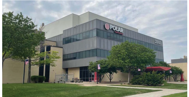
Construction is already underway on an expansion at Polar Semiconductor's manufacturing facility on Old Shakopee Road in Bloomington.
